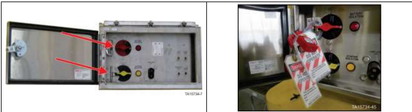
Battery isolation switch in OFF position with locks in place
